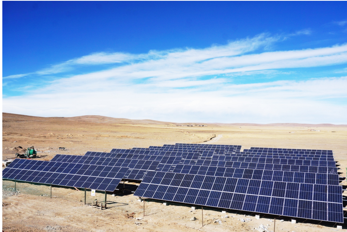
Solar Station System
